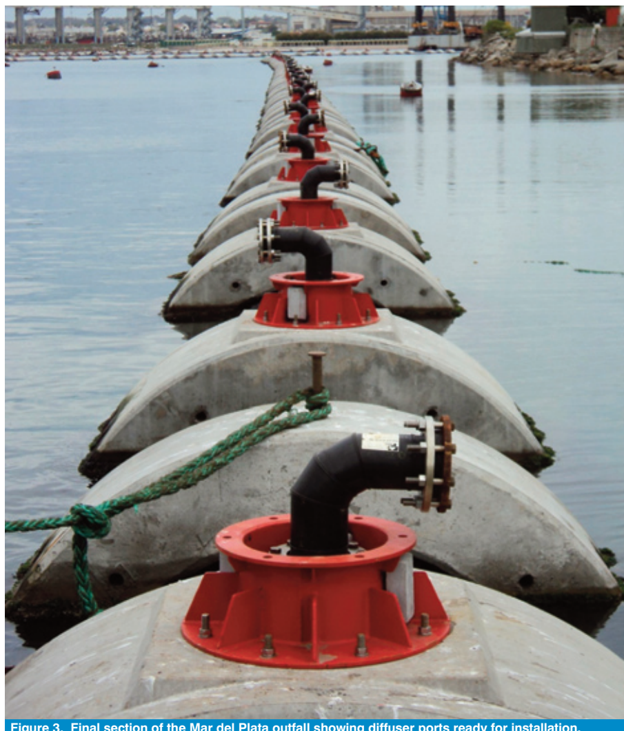
Figure 3. Final section of the Mar del Plata outfall showing diffuser ports ready for installation.
